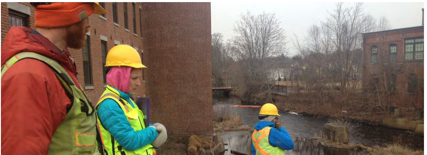
Nick, Candice, and Mike on site during construction of the Marland Place Dam removal.
