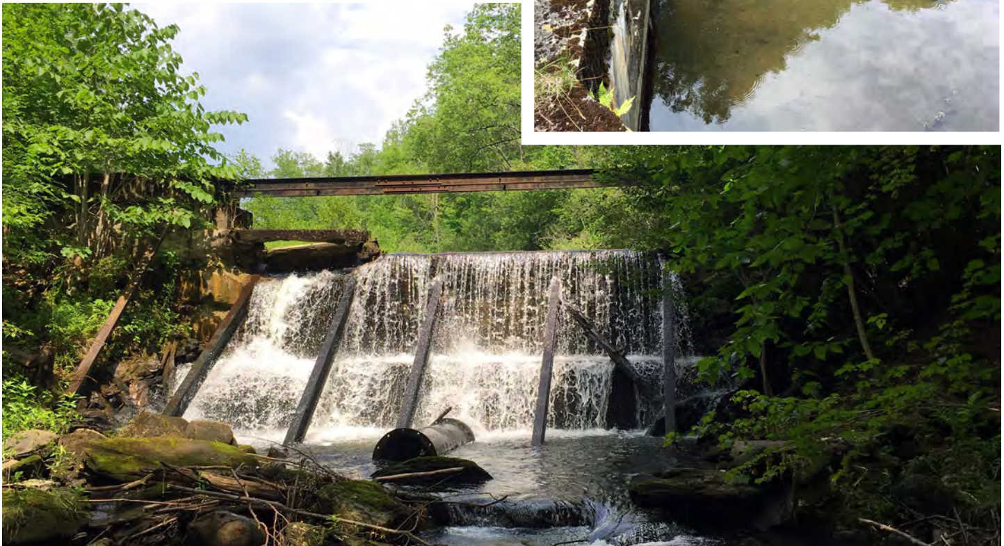
Top: Sediment build-up behind the dam wall. Bottom: Current state of the East Putney Brook Dam.
